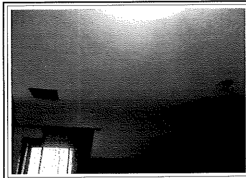
Exposed wiring and missing exhaust fan
