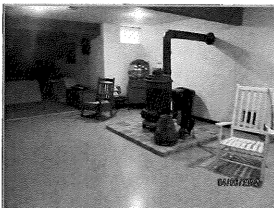
WOOD STOVE IN BASEMENT
