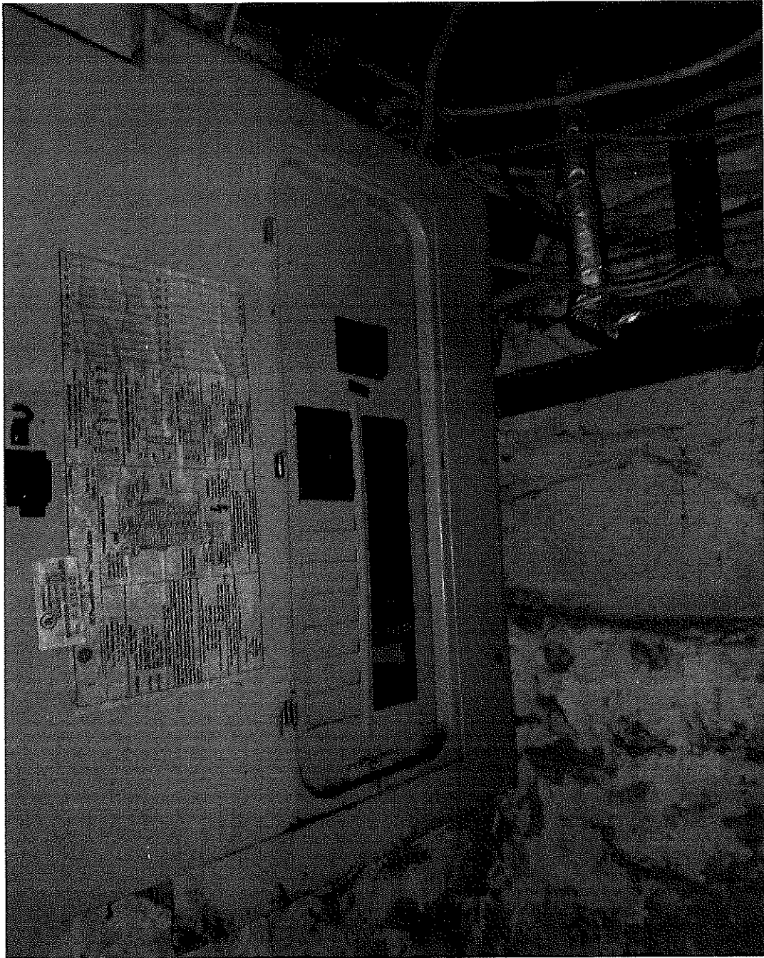
Outdated electrical box.
