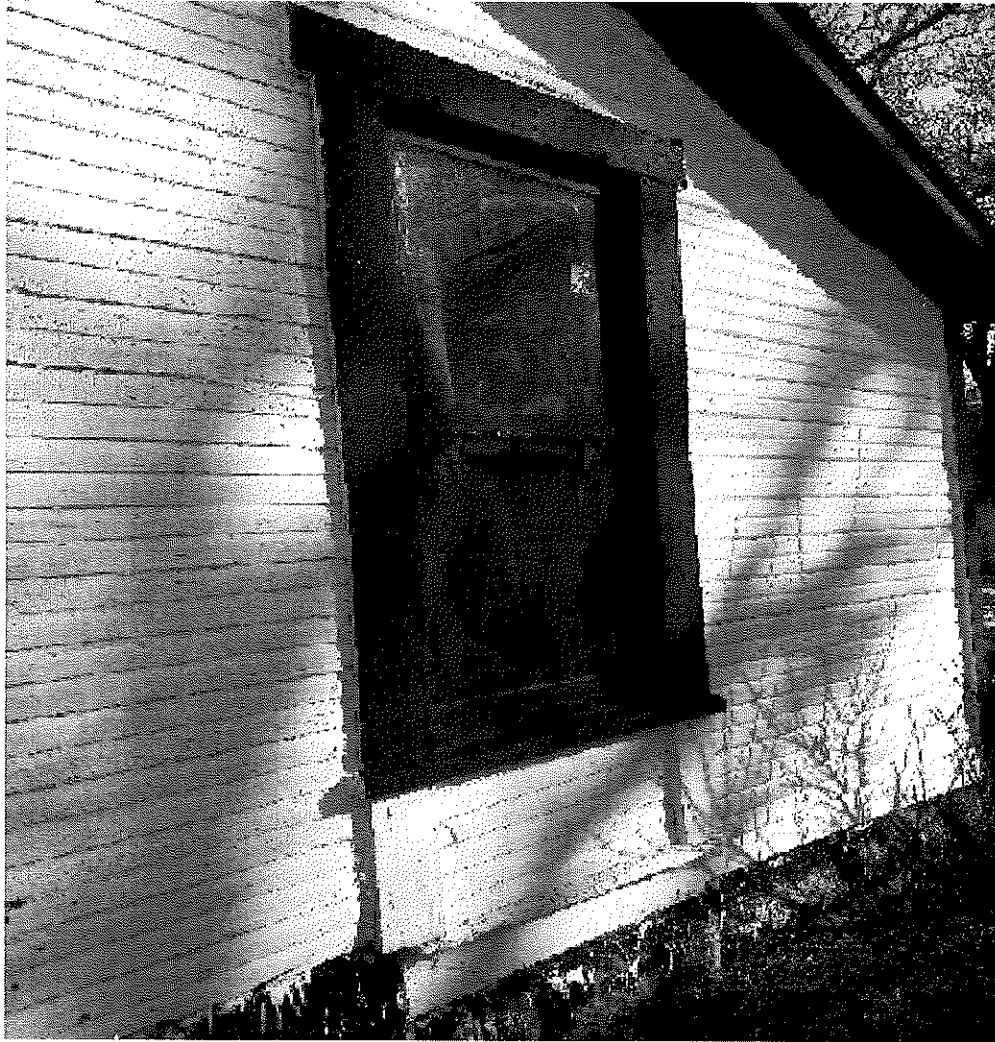
Original windows / frames are rotten. Covered with plastic and sealant.
