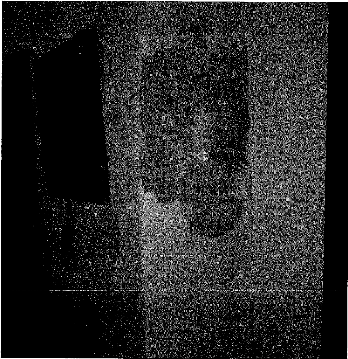
Bedroom chimney plaster falling off due to leaks around the exterior chimney.
