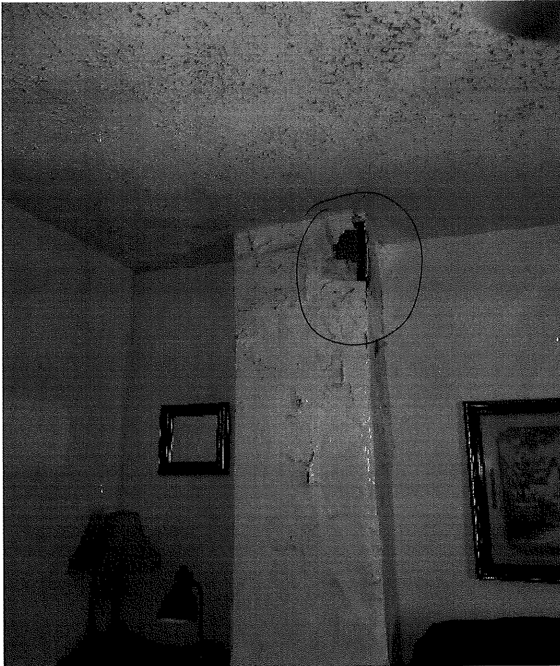
Living room chimney plaster falling off due to leaky chimney.
