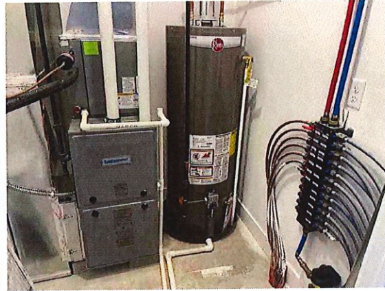
HVAC system/Water Heater
