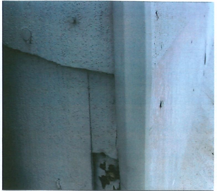
OUTSIDE SIDING DAMAGE
