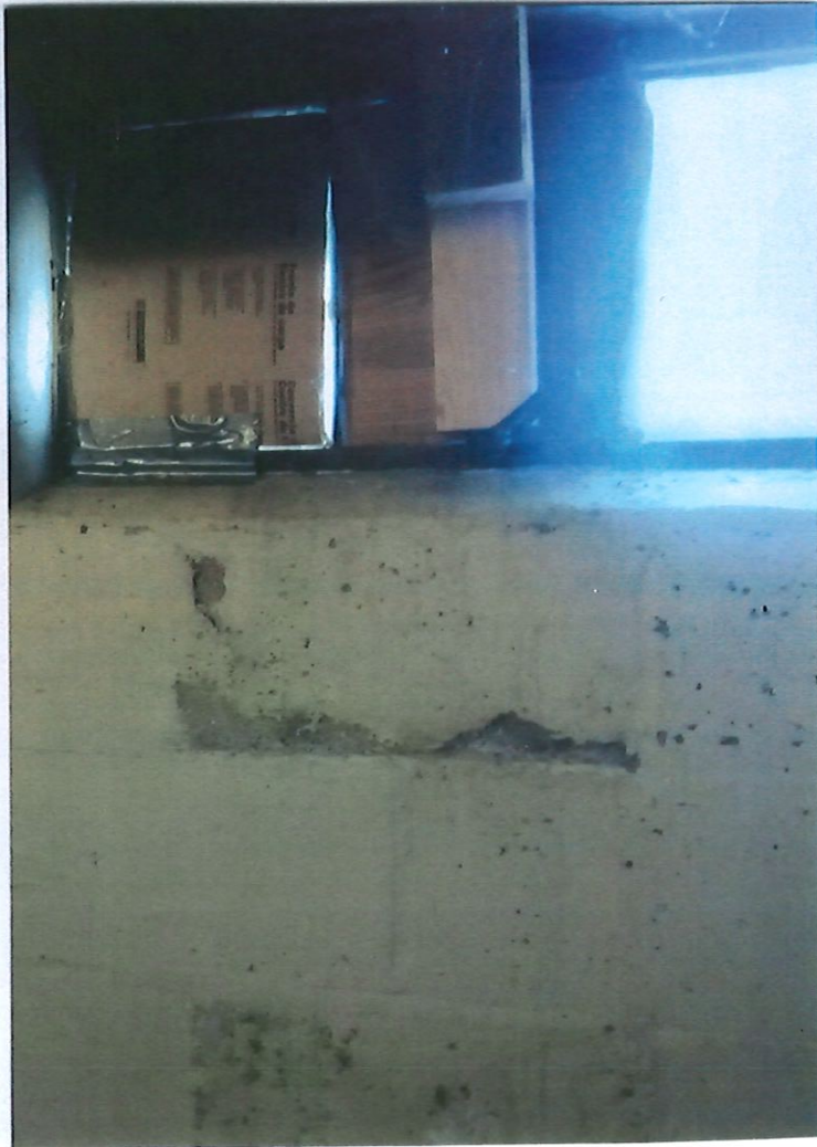
BASEMENT WINDOW BROKE OUT
