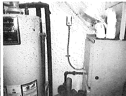
WATER HEATER / FURNACE
