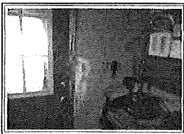
Exposed wiring at switches
